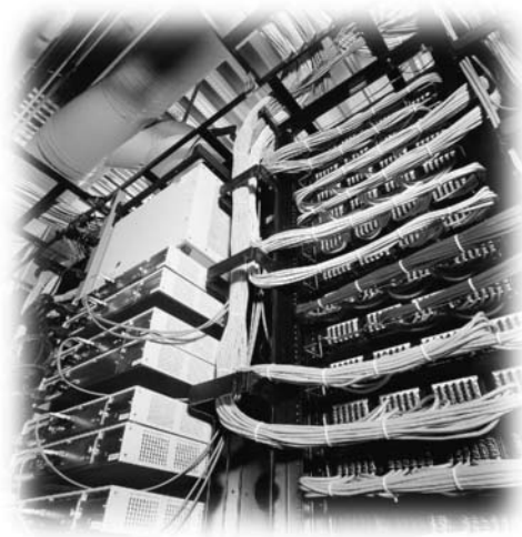
FIGURE 18.4 Lucent SYSTIMAX GigaSPEED Installation, rear angle view of patch-panel rack. (Copyright © 1999, Lucent Technologies, used by permission.)
